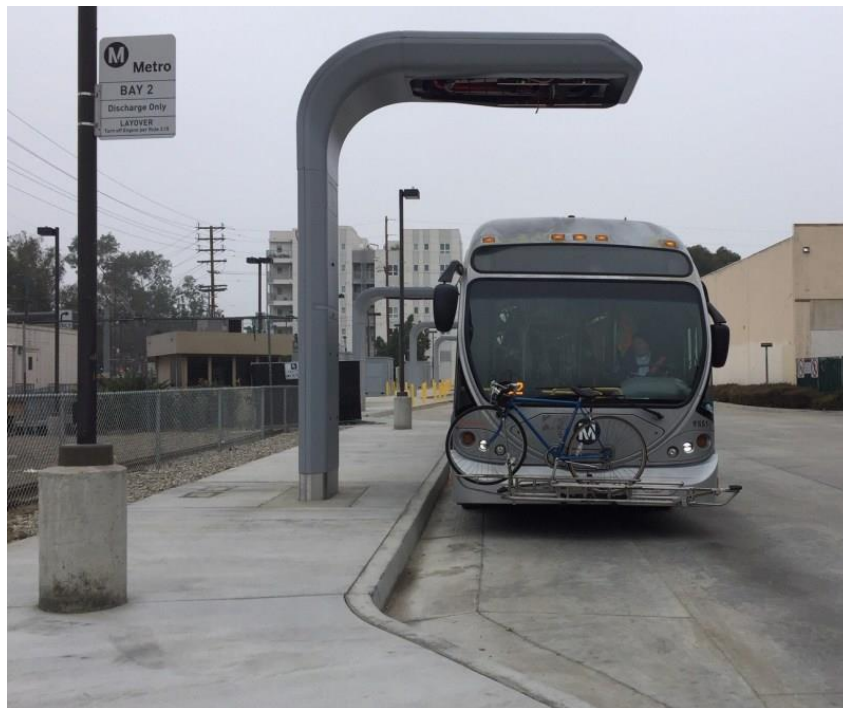
Figure 4-4. North Hollywood Station On-Route Charger
